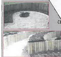
Example of 'Log Roll' Material being used in a retaining raised planting beds feature:- This material is suggested for the main structure of new DDA compliant ramped access.
